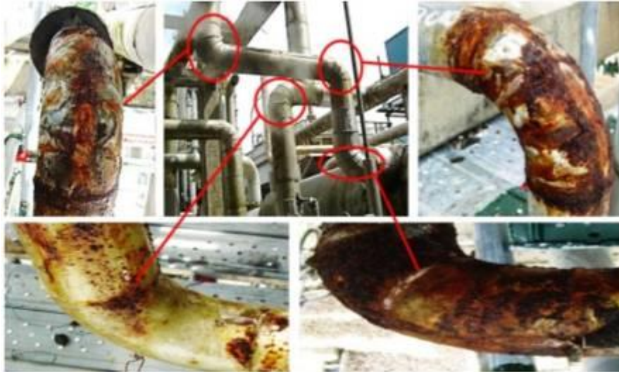
Fig 2. Corrosion Under Insulations [19]
