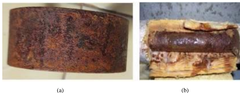
Fig 7. Corroded pipe under uniform corrosion type insulation (a) Result of research ; (b) Sulardi Research [26]
